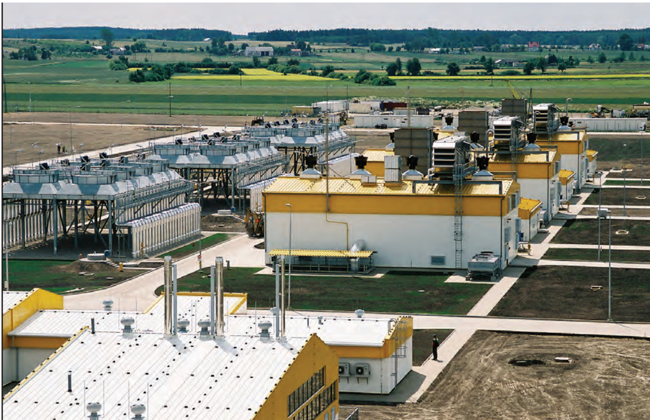
■ The recently inaugurated Ciechanow compressor plant in Poland has three SGT-600 compressor units installed. In Poland, there are 16 SGT-600 compressor units installed.
