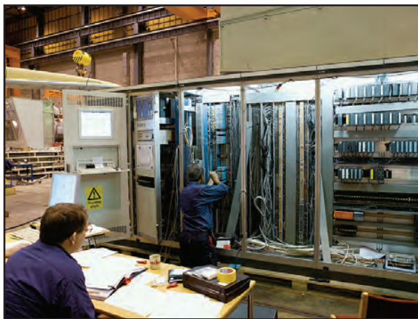
■ Testing is completed before shipment of the SGT600 turbine instrument and control panels (left) and UMD and UPS system (right).
